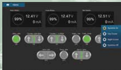
CZone Control & Monitoring
